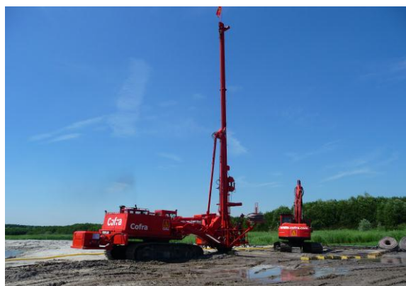
Figure 5. Installation equipment vacuum system
